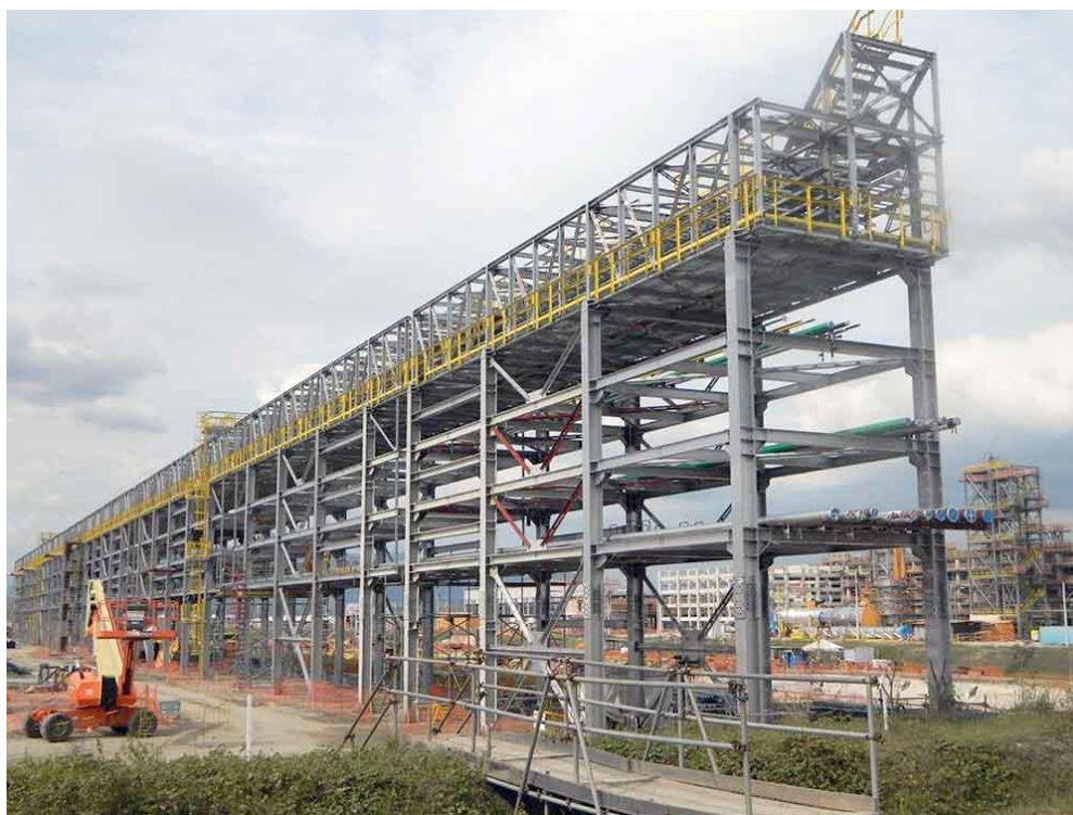
Figura 1 – Pipe Rack – COMPERJ - Petrobras
