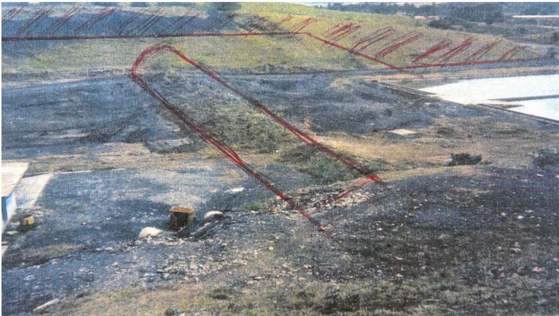
Photo 6.3 – Indication of lowering of the hill and construction of the dike. Source: GONÇALVES (2001).
