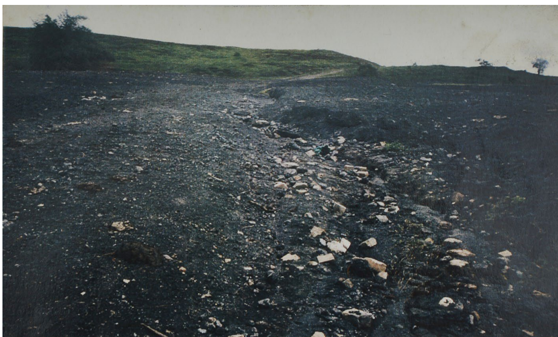
Photo 6-4. Erosion developed by surface water in the center of the slag dam carrying particulate material towards the Subaé River.
